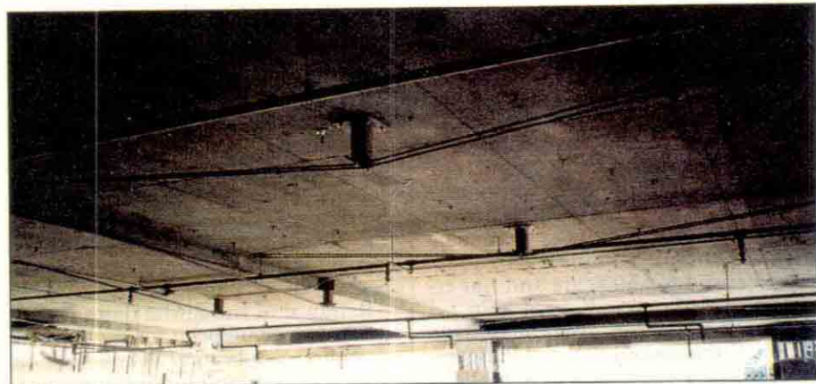
Post-tensioned cables were added to counter bending in slab after columns were cut for roof lifting.
