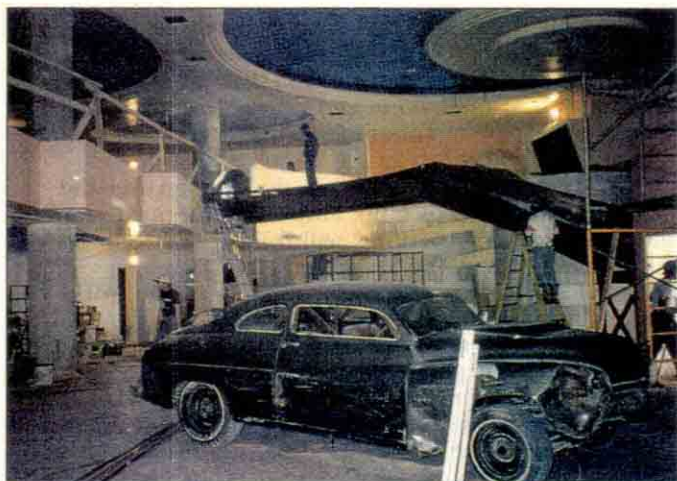
Movie auto had to be moved in early. Slab was cut to open up lobby area.
